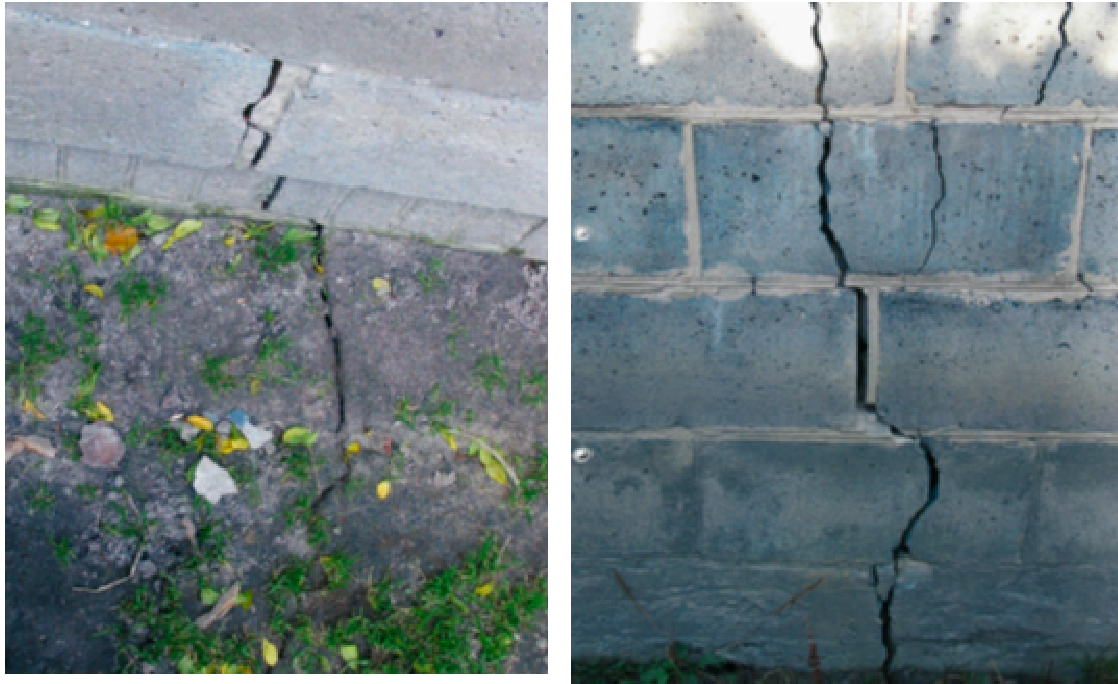
Fig. 4 Fissures that have occurred on the surface sequentially in zone 3.
